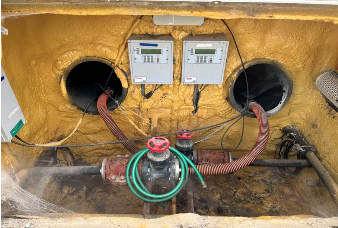
Photo 8 Display screens and leachate pump riser pipes. 11/5/2021
